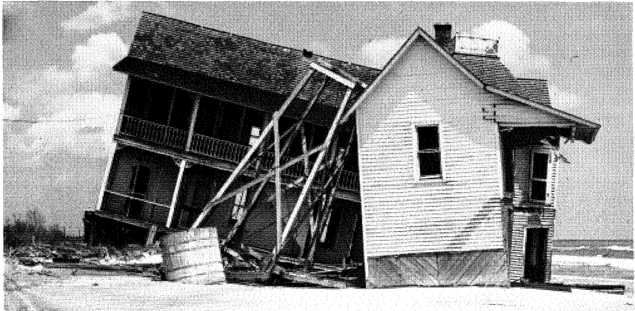
FIGURE 178. View of Wallops Island Association clubhouse on north end of the island, showing damage from erosion and storms, May 1949.
